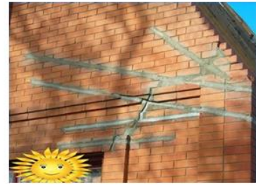
Crack in newly built brick wall
