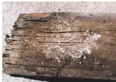
Wood destroying fungi
