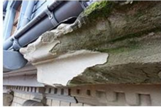
Wrong material used
