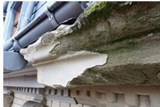
Wrong material used
