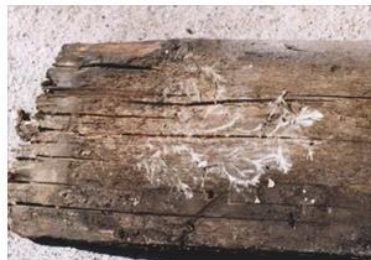
Wood destroying fungi
