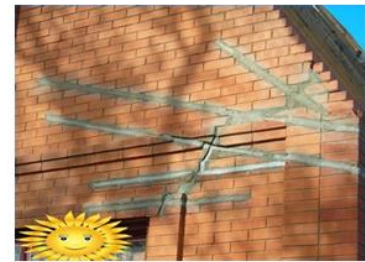
Crack in newly built brick wall
